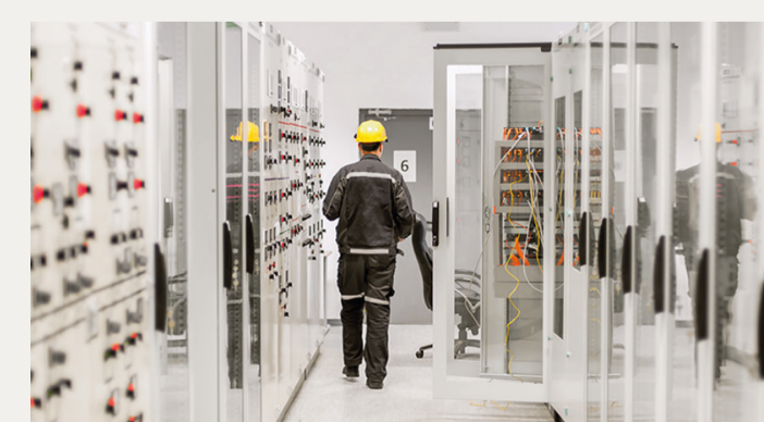
Electrical switching rooms
